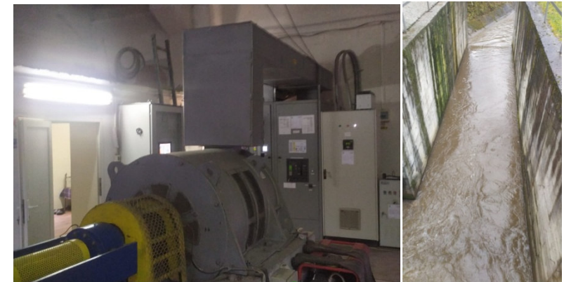
Micro-hydropower plant on the river Barnar – the electrical generator, the calming and escape channel
