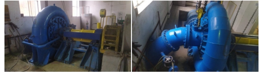
Micro-hydropower plant on the river Barnar – Francis turbine details; water discharge from the turbine
