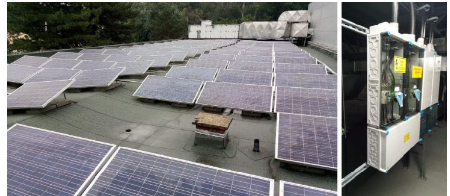
Part of the PV installation on the roof of Building B and some of the switch boxes and inverters
